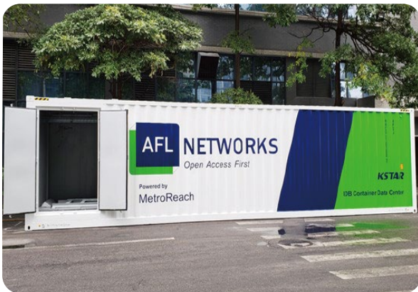
Container data center in Nigeria
