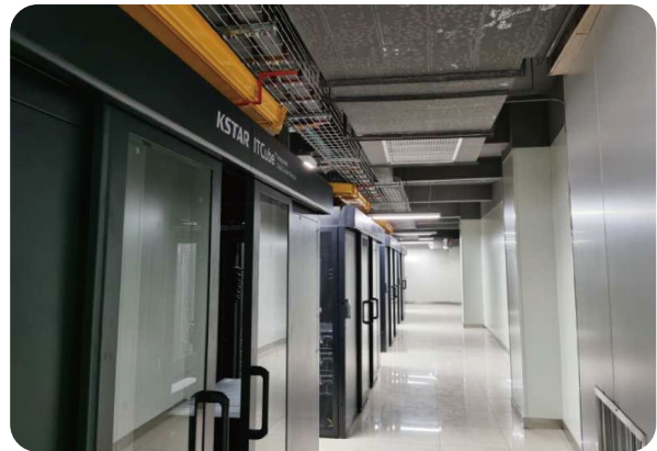
A data center in Jiangyou, Sichuan Province
