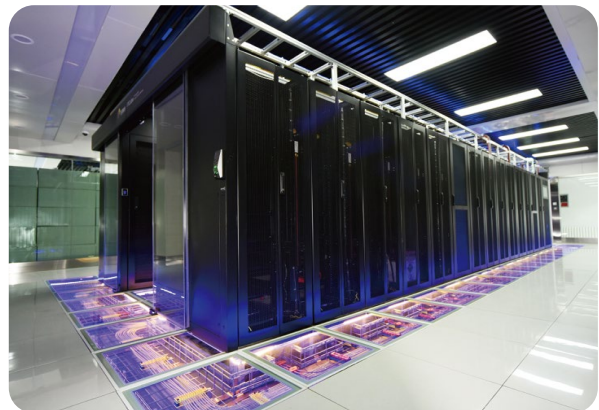
An enterprise data center in Gansu Province
