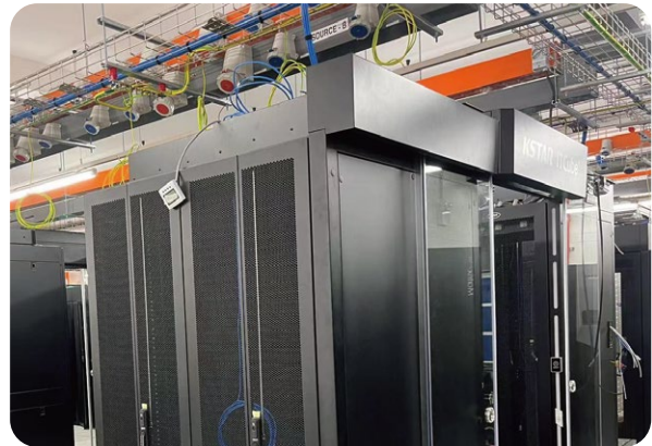
An enterprise datacenter in Singapore
