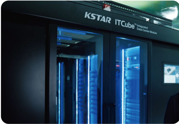
Malaysian Prime Minister's Department Data Center
